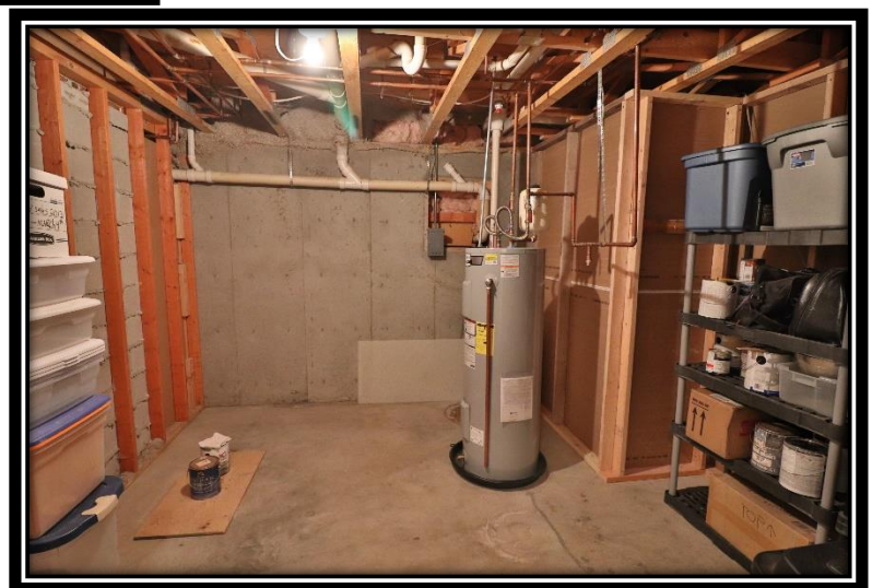
Utility Room Plumbed for a bathroom
