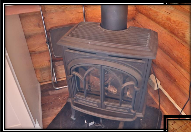
Propane Stove in Dining Area
