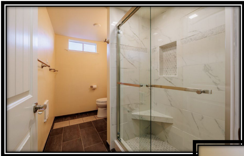
\frac{3}{4} Bath in Basement New Shower, Toilet & Plumbing New Vanity w/Quartz Countertops New Ceramic Tile Floor
