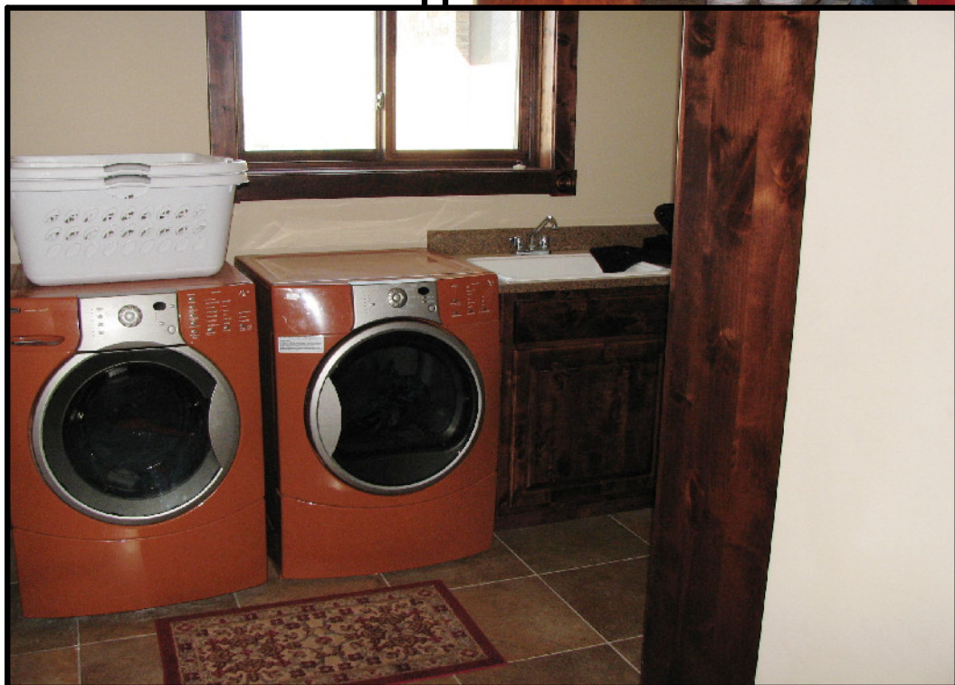
Laundry Facilities with Utility Sink
